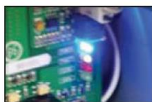
BOARD POWER ON LED SIGNAL CHECK
